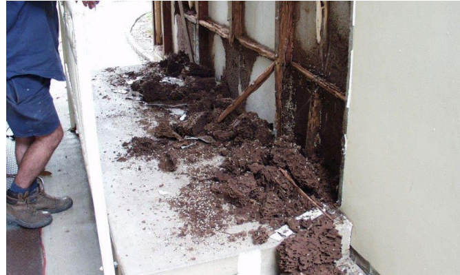
Termite damage can cause a financial burden
