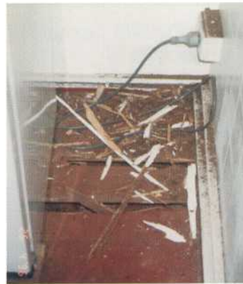
Termite damage. Beyond repair - don't let this happen to you.
