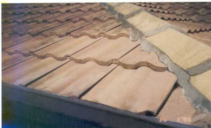
The same roof another year on. The algae started to reappear lightly in late 1997.
