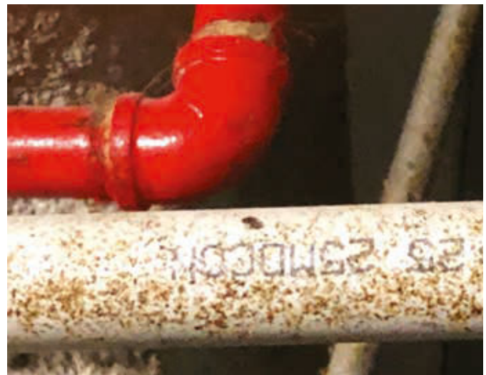
Flies and spotting (droppings) present on an electrical conduit
