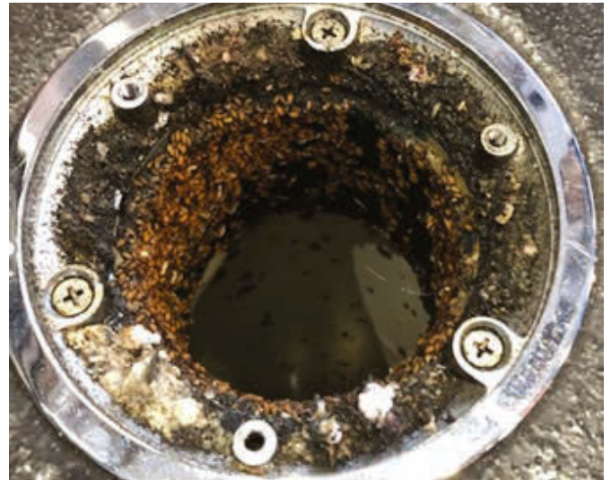
Floor drain opened for inspection of potential fly breeding ground.
